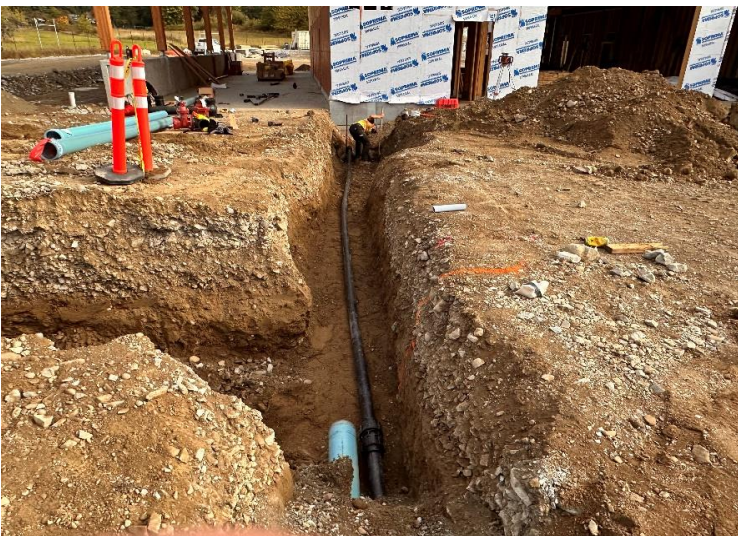
Water Connection to Building
