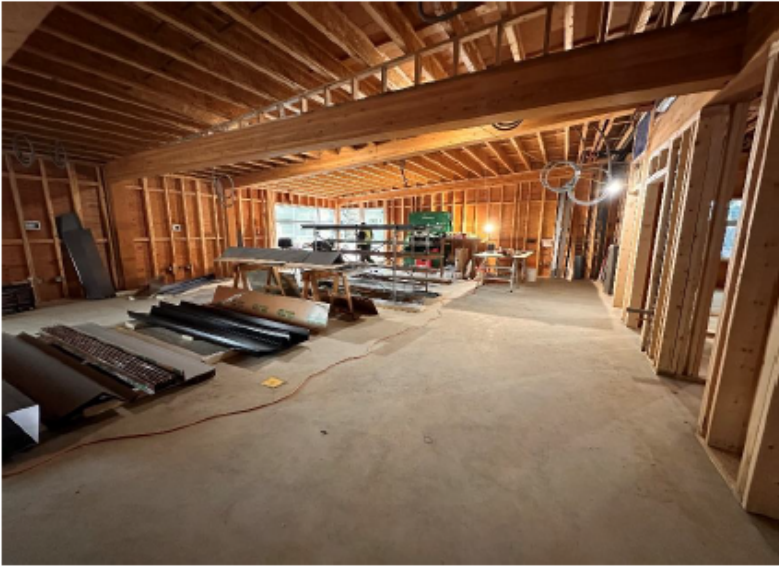
Temporary Shop in Traing Room
